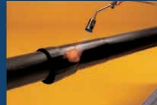
Shrinking of the joint.
